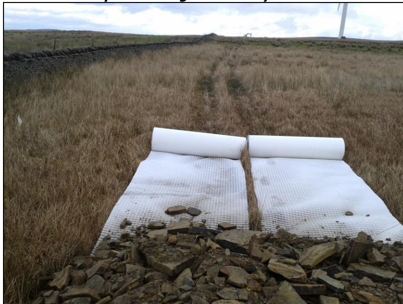
Plate 13: semi-permeable geotextile layer
