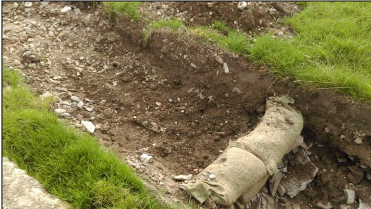
Plate 4: Typical check dams - to be installed in drainage ditches adjacent to the new spine road
